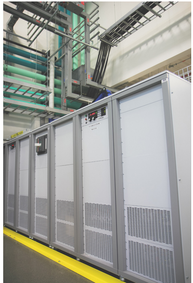
1.5 MW solar array emulator using Magna-Power MT Series power supplies at the National Renewable Energy Laboratory in Golden, Colorado USA
