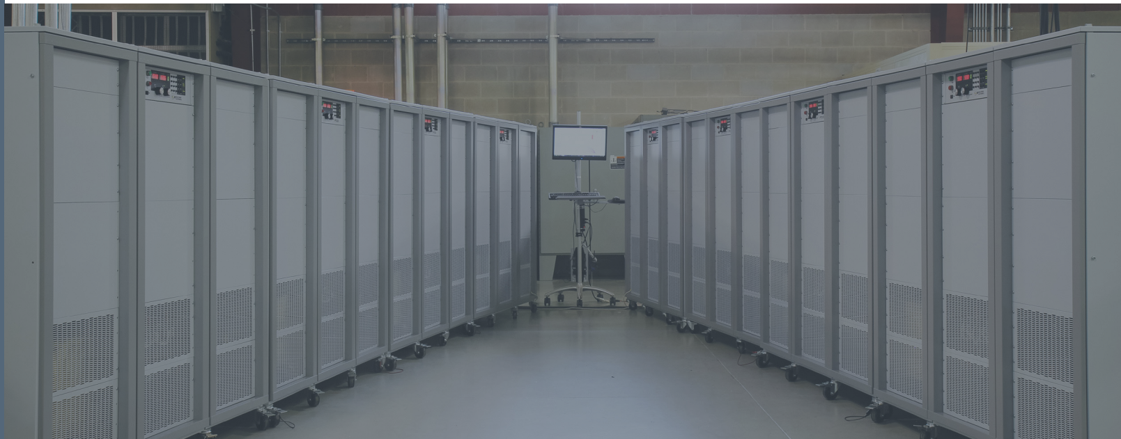
Qty (8) 250 kW MT Series units in master-slave parallel to form a 2 MW system
